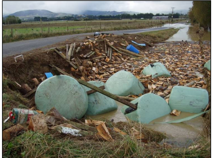
Floatable farm debris block a culvert
