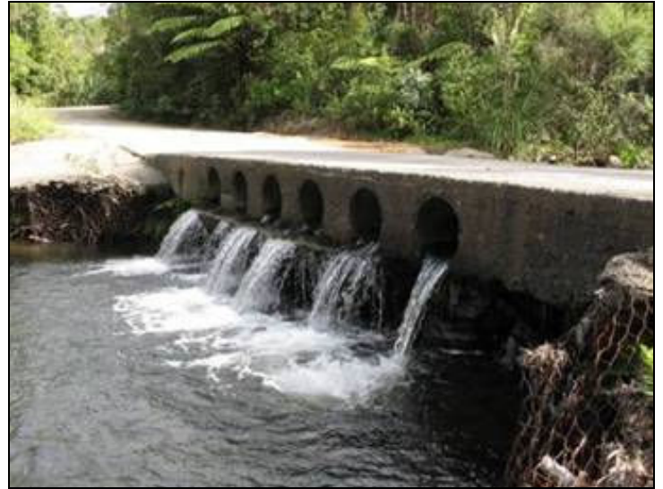
Perched culverts present a barrier to fish passage
