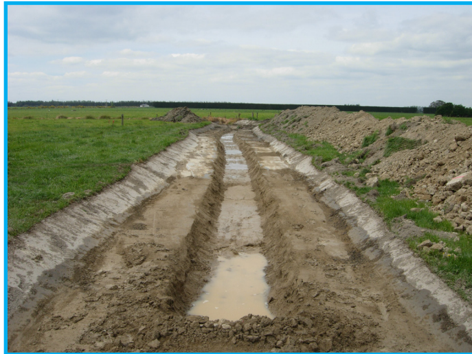
Photo 1: Artificial two-stage channel in a newly-constructed drain. The floodplain levels were set to allow for floodwaters to surpass onto the banks where sediments could settle out. Grass and tussock plants on the floodplain bench enable further nutrient cycling.
