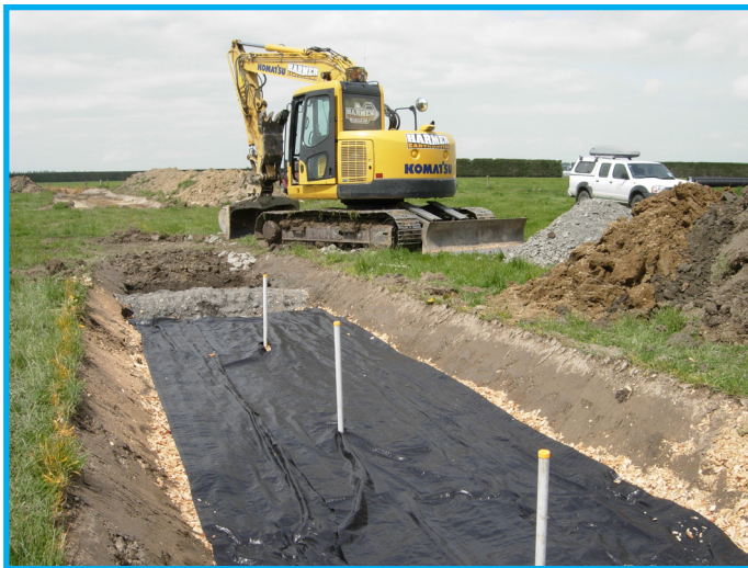
Photo 2: In-stream denitrification bioreactor. Woodchips line the bottom of the new drain to encourage nitrogen removal via denitrification. Monitoring wells were also installed to allow for ongoing monitoring within the bioreactor.
