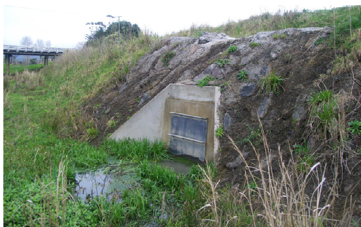
Recessed headwall and floodgate
