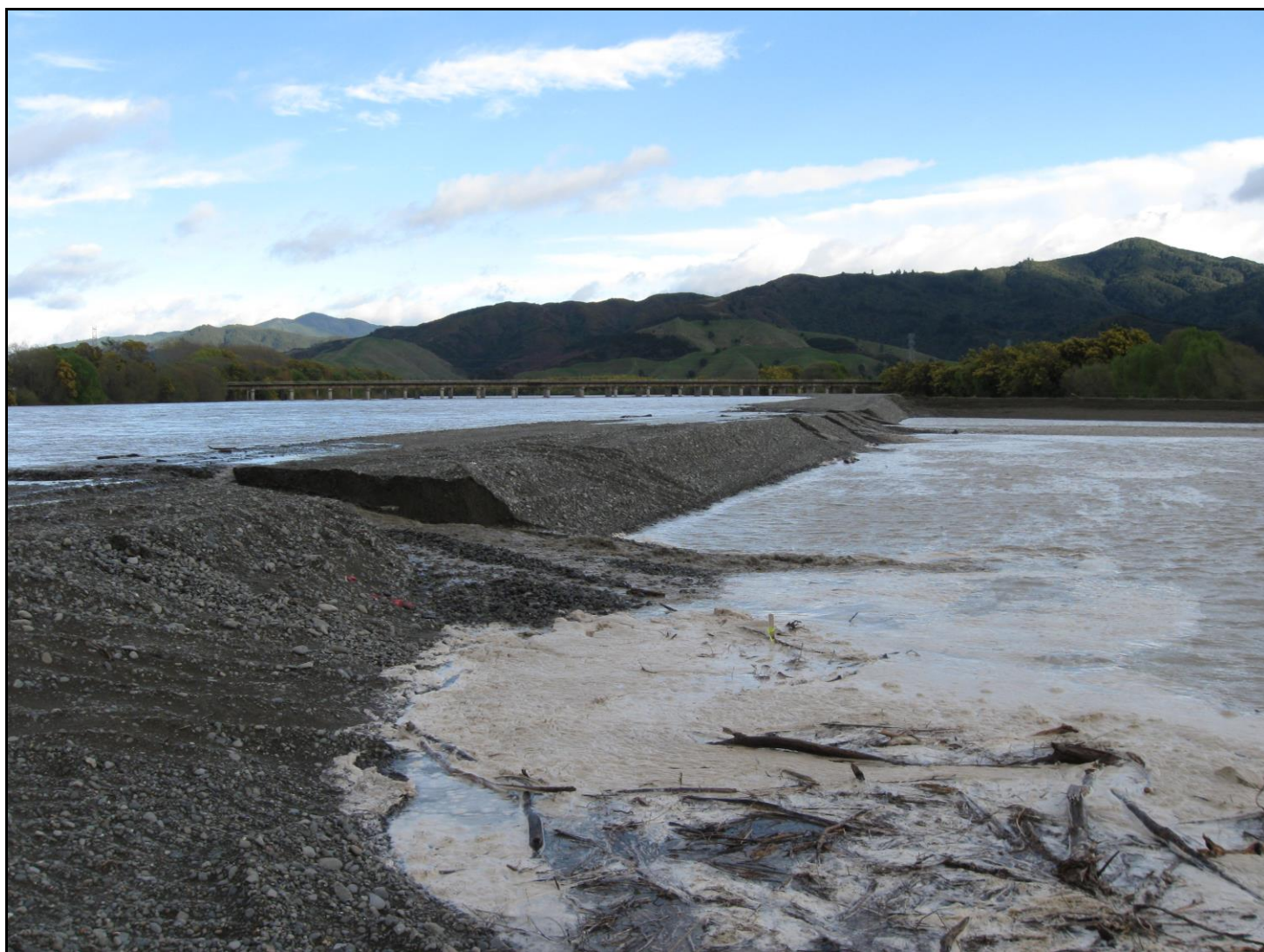
Looking upstream at the Erodible Bank just as flood waters are beginning to breach the Fuse Location
