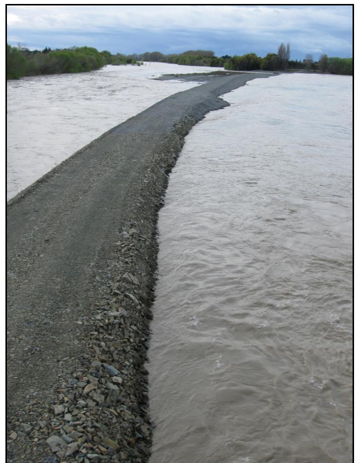
The Wairau Diversion's Erodible Bank looking downstream to the head of the Wairau Diversion
