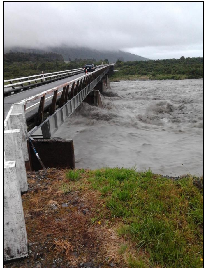
Wanganui Bridge looking west after the pier-underpinning work in 2010 and just prior to the abutment washout in January 2013
