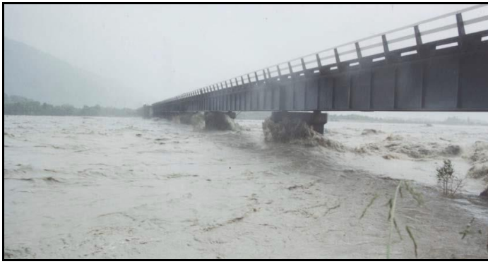
Wanganui Bridge looking downstream during a large flood in December 1995 (Photograph by M Shearer, WCRC Engineer)
