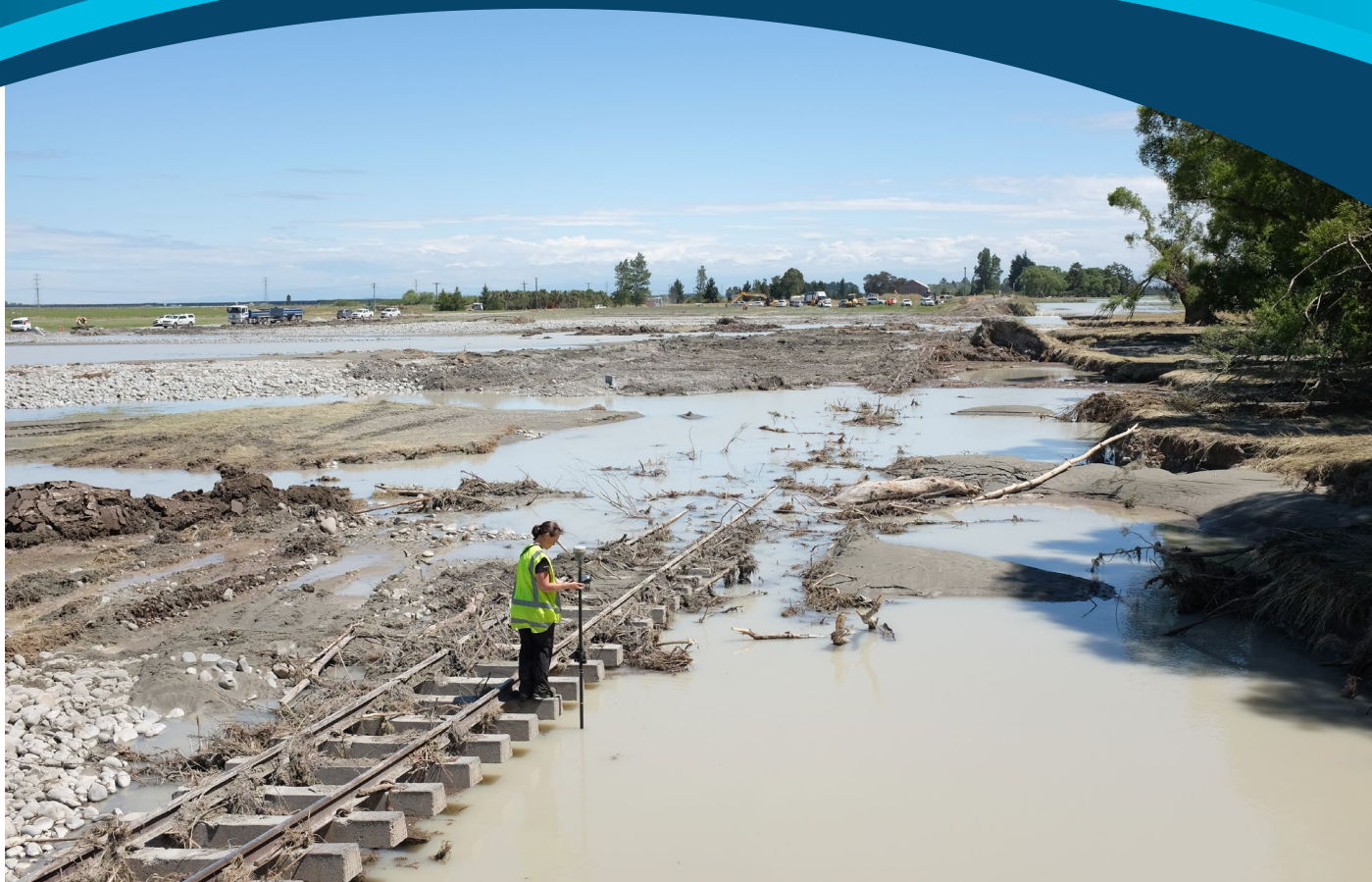
Destruction of railway track, outside of the permitted Rangitata river channel during December 2019 flood (Jochen Bind, NIWA).
