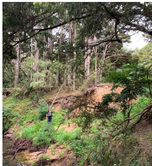
Figure 1 - Large bank failure on the Kourawhero Stream - Scott Speed for size reference
